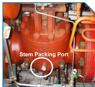
Gas Leak Isolation
