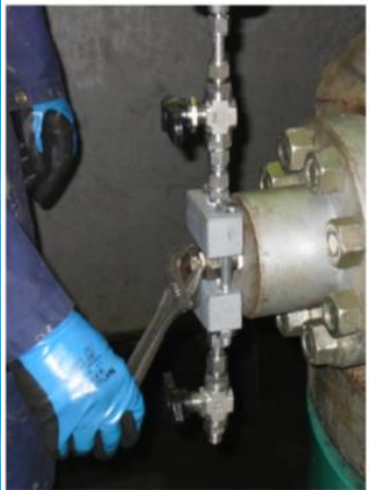
500psi Locked In The Clamp Assembly Back Out The Bleeder Screw
