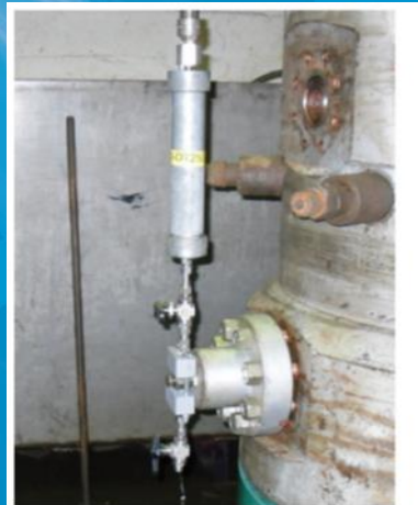
Mac-Pac Cylinder Installed
