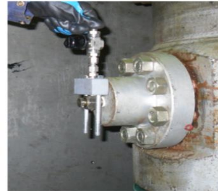
Leak Path Present Top Clamp Assembly Valve Closed
