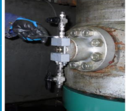
Leak Path Present Bottom Clamp Assembly Valve Open
