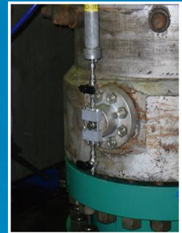
Bottom and Top Valves Closed
