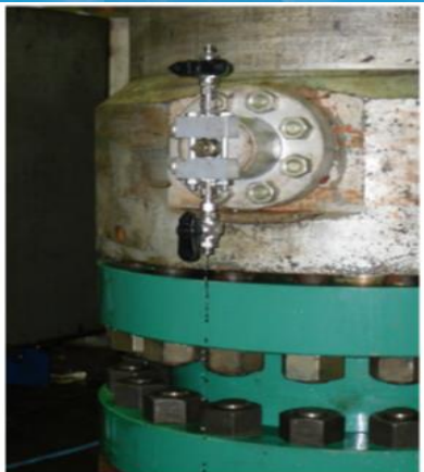
Clamp Assembly Installed Pressure Leak Deflected Downwards
